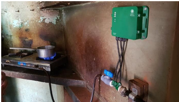
Figure 2: Biogas meter for remote monitoring.
