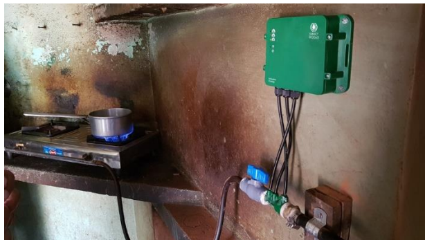
Figure 2: Biogas meter for remote monitoring.
